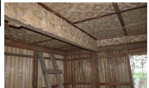
View G abuilding. Note ceiling & walls.
