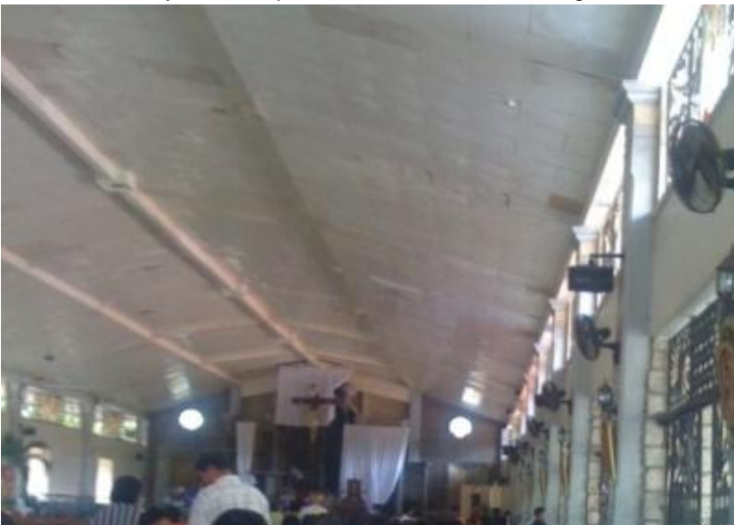
The "Present" view a few weeks ago during a wake at the side altar. The main altar was undergoing repairs for another project hence it was not used. Note cloth drapings at far end. The photo does not do justice to the actual ceiling condition: warped ceiling tiles, water stains on the paint, and a general decrepit look. One of the local civil engineers here, Joel Borromeo, told us that the roof structure has probably moved, hence all the water leaks during heavy rains. It wasn't that way before.
